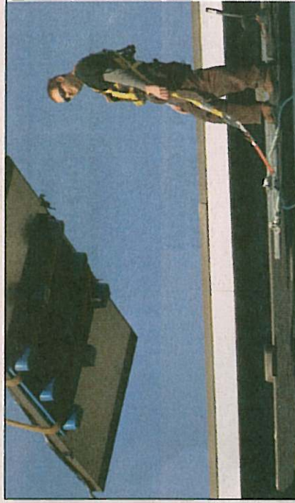
Don Denton/News staff Nathan Dockstader, Pacific Solar Smart Homes, watches as a crane lifts a solar panel for domestic hot water heating on to the roof of Patrick Chénier's house.
